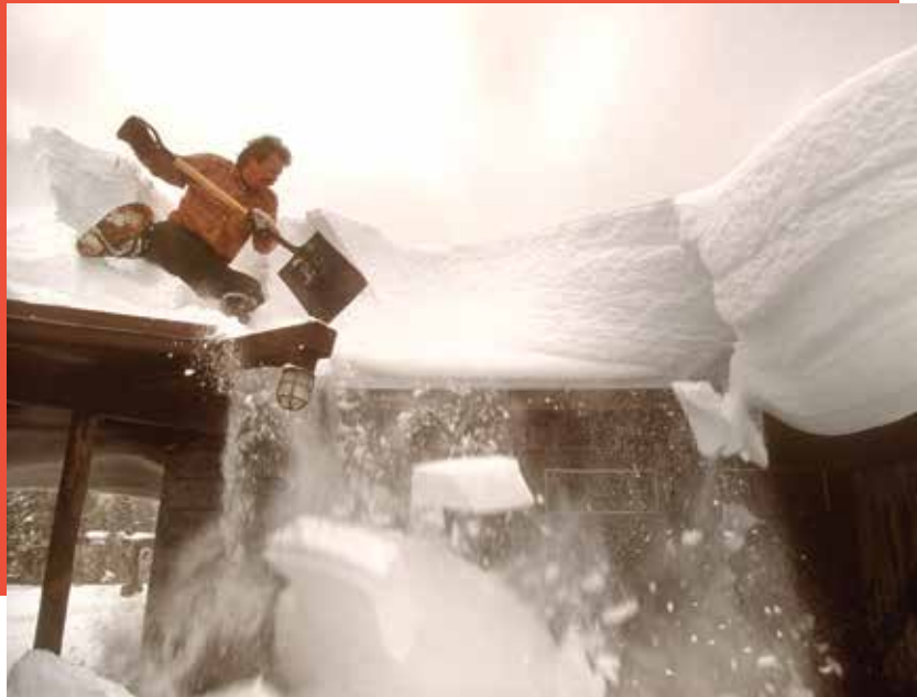
Getting it done, circa 1999. Fuller winterkeeps approximately 100 buildings in Yellowstone's Canyon Village area, where average winter snow depth ranges from 3-6 feet. PHOTO BY JEFF VANUGA
